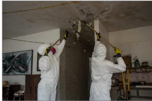
AmeriCorps members work to repair homes damaged by Hurricane Maria in Humacao, Puerto Rico.
